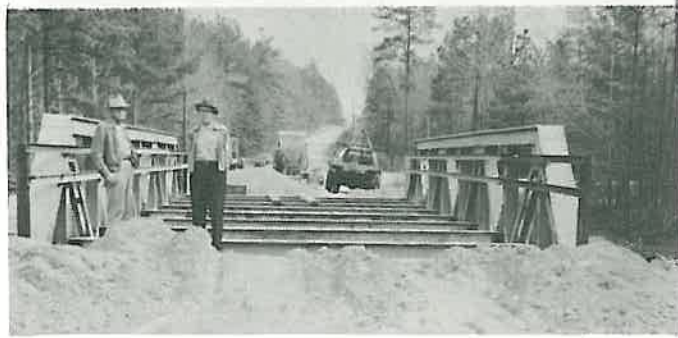
According to W. E. Hicks, engineer of District 7 engineer, “old steel never dies,” as evidenced by the two pictures he sent, shown here. A salvaged steel truss was used to replace a single lane untreated timber bridge on a Milum Act road, Mt. Holly to Smackover, Route 160, Section 5, in Union County.
